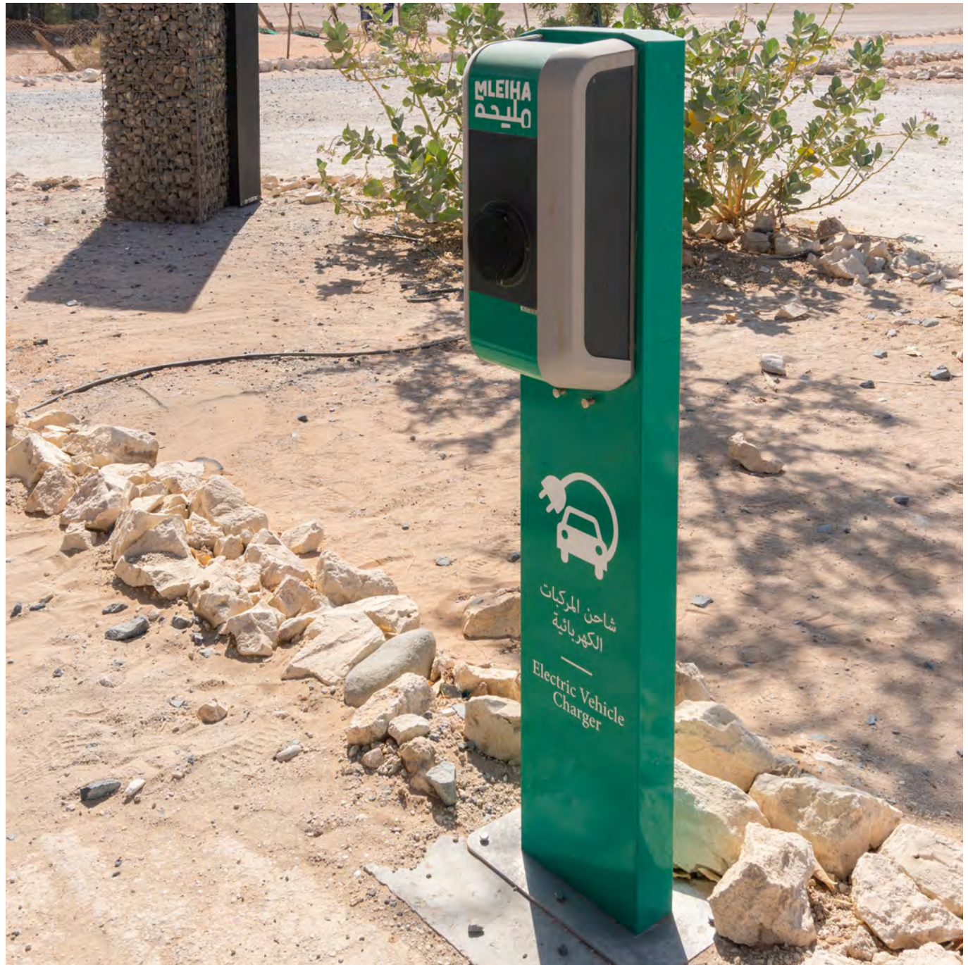
Example of EV charging station
